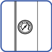
1. Should be completed in the morning or when the boiler is cold with zero pressure.
